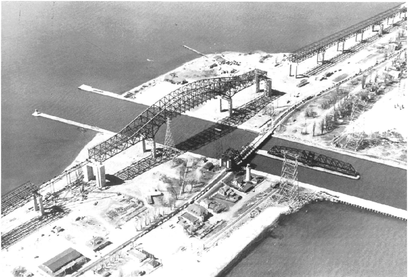
Figure 7: Paradise Lost?: the construction of the first Burlington Skyway Bridge, 1958, which was opened to traffic later the same year. Source: Broe's Studio. Courtesy of Dominion Bridge Company Limited, National Archives of Canada, PA-138903.
