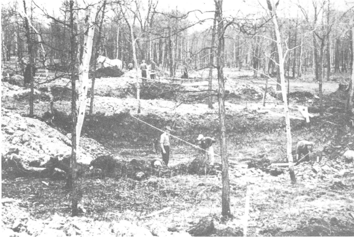
Figure 5: Bird Construction Company workers carefully excavate around existing mature trees to preserve the woodland. Prefabricated house walls were constructed and stored off-site for eventual on-site assembly via “cranemobile”. (Photo reproduced with permission of Wildwood Park History Book Committee)
