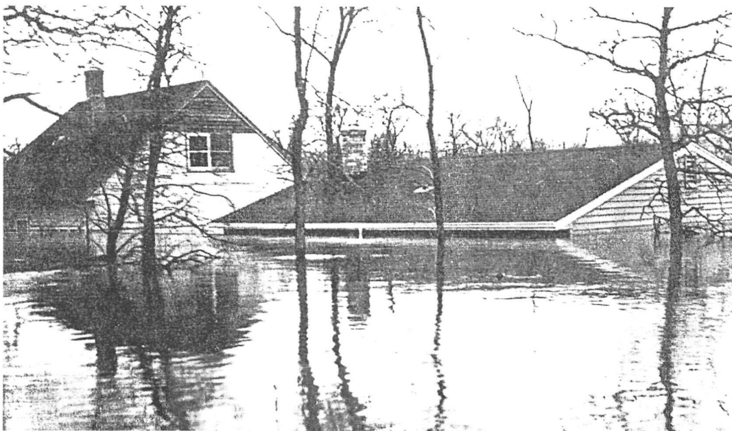
Figure 7: Many homes were flooded to the level of first-floor ceilings in 1950. While all homes were severely damaged, none were destroyed, and most were substantially restored by later that year. (Photo reproduced with permission of Wildwood Park History Book Committee)
