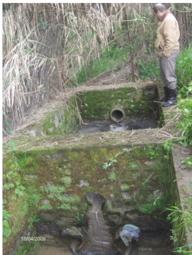
Figure 2. Bassin de filtration au village Tala Bounane (Tizi Ouzou). Filtration basin in Tala Bounane village (Tizi Ouzou).
