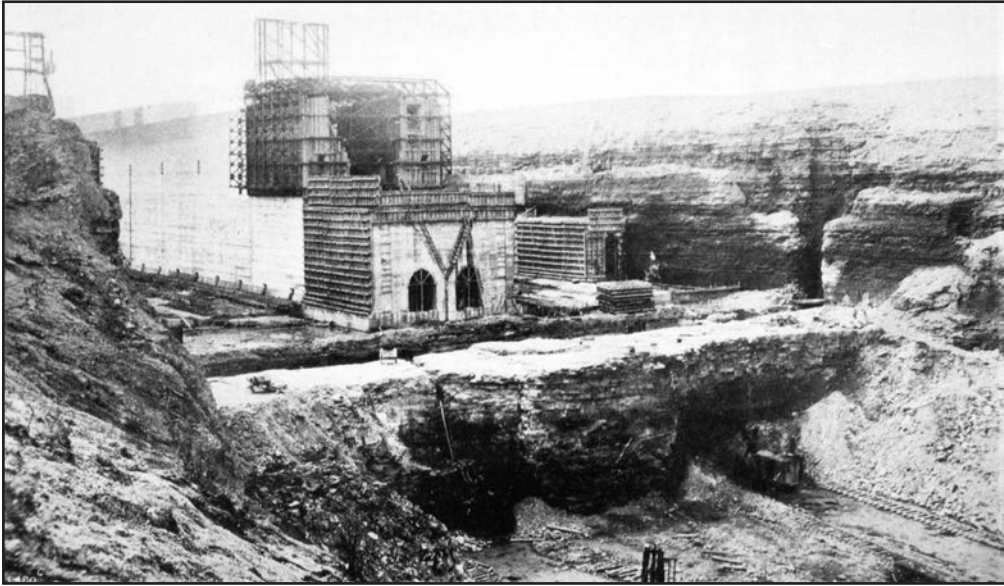
Thorold, Ont. c. 1925: construction of the paired flight locks, revealing the width and depth of the excavation and the size of the monolithic lock chambers. A locomotive is on a track on the lower right. (P.J. Cowan, The Welland Ship Canal Between Lake Ontario and Lake Erie 1913-1932 , London: Offices of Engineering , 1935, 42.)
