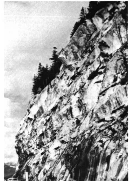
Figure 3 A high rock slope in granitic rocks north of Vancouver which has been undercut by a transportation route. Many joints are parallel to the original surface and individual blocks occasionally break loose in rock falls.
