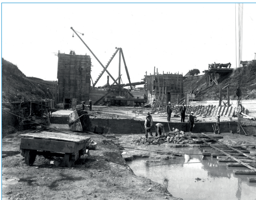
FIG. 6. PREPARATION WORK FOR ST. ANDREW'S LOCK AND DAM, LOCKPORT, MANITOBA. H. E. VAUTELET (DESIGN ENGINEER), 1900–1910, PHOTOGRAPHED IN 1908. ARCHIVES OF MANITOBA PHOTOGRAPH COLLECTION. 1984-129. LOCKPORT 28, CONSTRUCTION, 1908, P1188, N17222.
