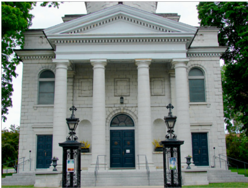
FIG. 37. ST. GEORGE'S CHURCH, RITUAL WEST FAÇADE, 1842; DETAIL OF STONEMWORK ON FAÇADE, PORTICO, AND STYLOBATE. | PHOTO: PAUL CHRISTIANSON, APRIL 2021.
