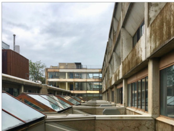
FIG. 14. VIEW ABOVE THE SKYLIGHTS OF THE STUDENT STREET LOOKING NORTH, MACKINTOSH-CORRY HALL (R.J. THOM ARCHITECTS, 1972-1974), QUEEN'S UNIVERSITY, KINGSTON. | JAMES ASHBY, 2019.
