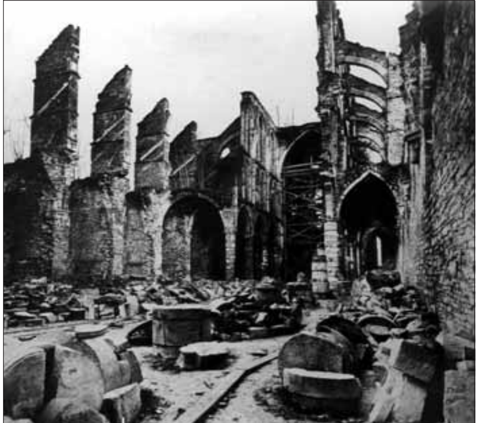
Ill. 5: The first stage of restoration consisted in cleaning the site and sorting the stones, which could be reused for anastylosis. Nave of the church, December 1893.
