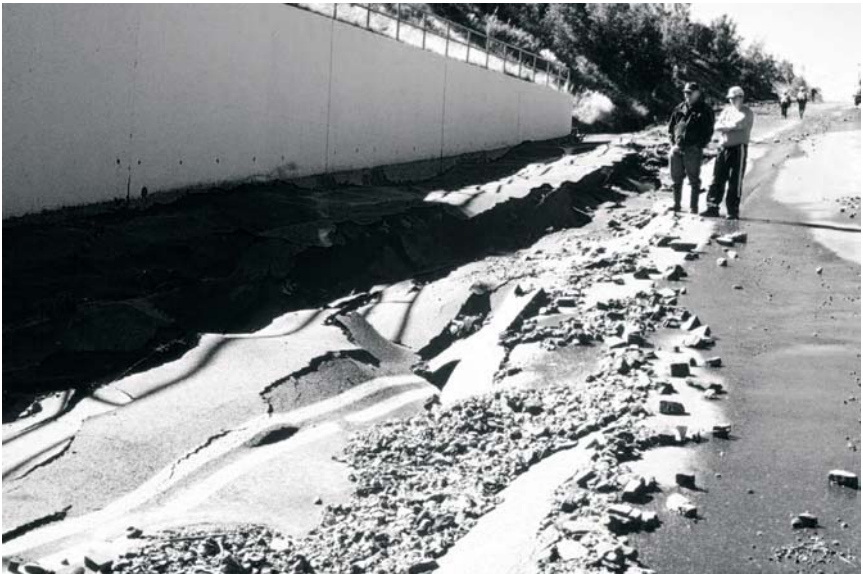
Figure 11. Flood damage on Shea Heights road, September 2001.
