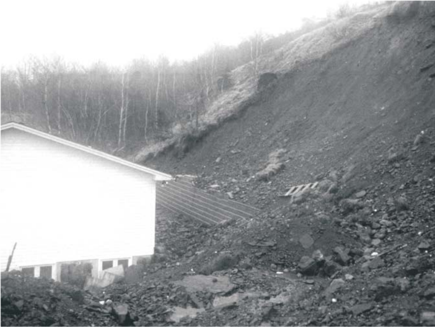
Figure 5. Recent construction on Southside Road, undercutting steep banks of till and increasing landslide hazard.
