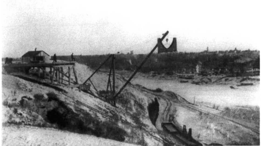
Figure 6 Siding from the Edmonton, Yukon and Pacific branch of the Canadian Northern Railway for the delivery of steel and stone for the Alberta Legislature. A five ton stiffleg derrick handed materials from the cars to a trestle and light railway on the top of the hill. To the southeast across the North Saskatchewan River the skyline of the town of Strathcona can be seen (Provincial Archives of Alberta, A 11017).
