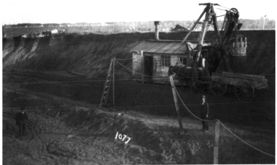
Figure 2 Steam-powered shovel excavating for the foundations of the Legislature (Provincial Archives of Alberta, B3354).
