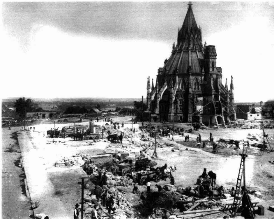
Figure 3 Preparation of Parliament Hill for reconstruction of the Centre Block, 15 August 1916. Workmen with horse teams are removing the last of the rubble from the foundations of the former building. In the middle ground, in front of the Library, another crew is drilling blast holes for foundation excavations. Only the Parliamentary Library remains intact. Its shored up entrance, which connected it to the Centre Block, can be seen beyond the drilling crew. National Archives of Canada PA130624.
