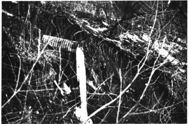
Figure 6 A) Bellamy Ravine, one of the most impressive of the ravines along Scarborough Bluffs. Its headward development and rapid downcutting have been aided by rapid urbanization of its catchment (Fig. 4) and uncontrolled storm runoff ( B )
