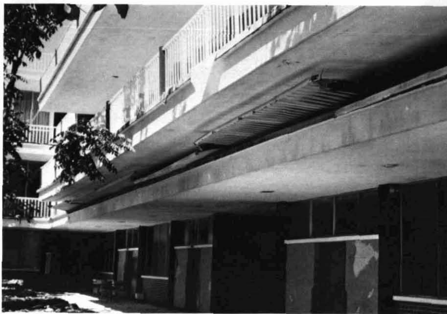
Figure 7 Collapsed second floor of a school in southeast Guatemala City, about 30 km from fault.
